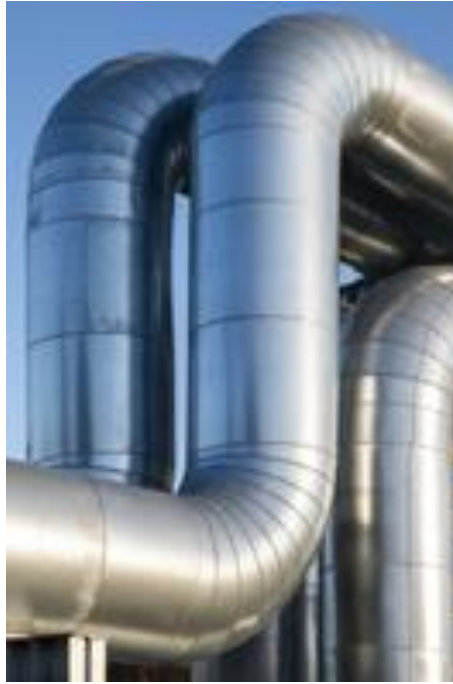
Figure 6.1-2. Exemplary picture of a steam pipeline.
